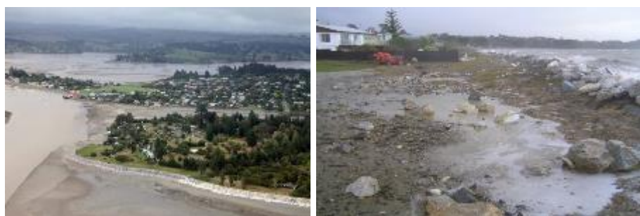
Figure A.6: Photographs at the Mapua foreshore (left) and Ruby Bay rock revetment after a wave overtopping event
