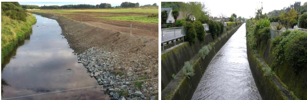
Figure 1. Two examples of river habitat modification; (left) bed lowering and bank contouring for land drainage and erosion prevention (respectively) in an agricultural catchment, and (right) bed lowering and concrete bank reinforcing to protect urban properties from floods.
