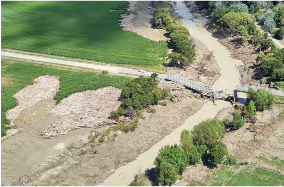
Figure 4: Broken State Highway 35 at Hikuwai
