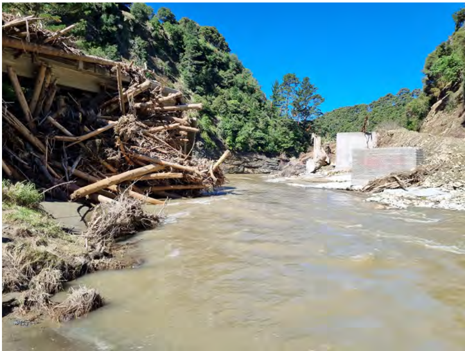
Figure 5: Broken State Highway 2 at Waikare
