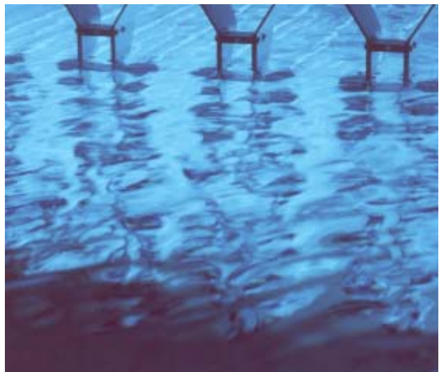
Water passing through the final stage of treatment (ultra violet light disinfection) at the wastewater treatment plant.
