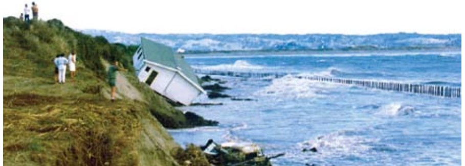
> Shaky Foundations: a house slides into the sea at Ohiwa Spit, Bay of Plenty. Photo: R.K.Smith.
